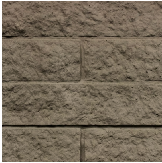
EXTERIOR CLADDING SPLIT FACED CMU: VWP-1B PAINTED 214E PMS 4231C MEDIUM BROWN
